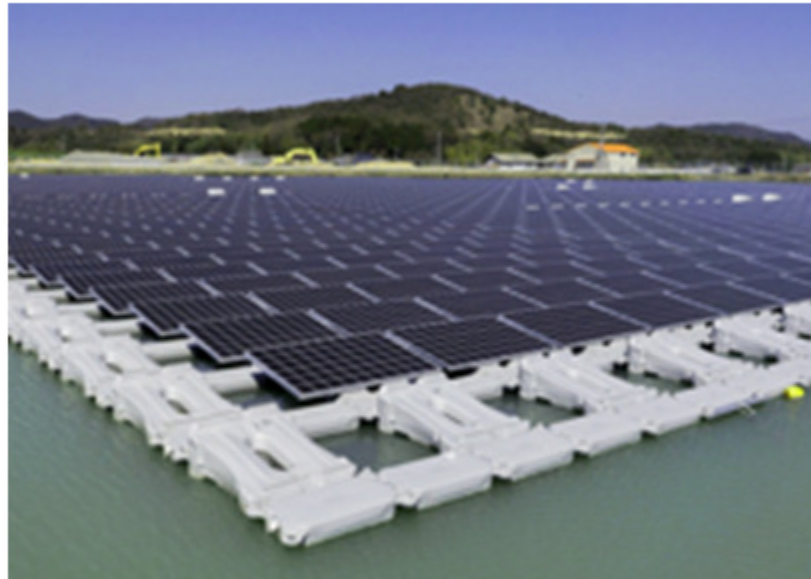
Figure 1 – Floating Solar PV Farm in Kato City, Japan
